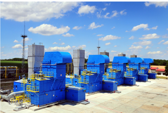
gas compressor station
